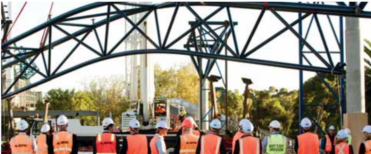
Top: The redevelopment works ensure the Australian Open will remain at Melbourne Park until 2036. Above: A milestone was reached as the final truss was installed on the Eastern Plaza in 2012.
